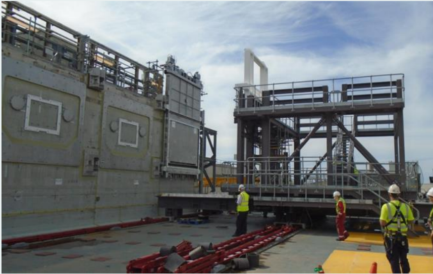
PFCS showing compartments four, five and six. The first Silo Door is installed onto compartment 6 with the DIF and East West Movement System visible
